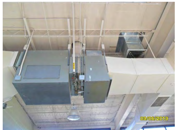
A-34. Administration Building, Assembly Hall, Room 120, Northeast HVAC Unit.
