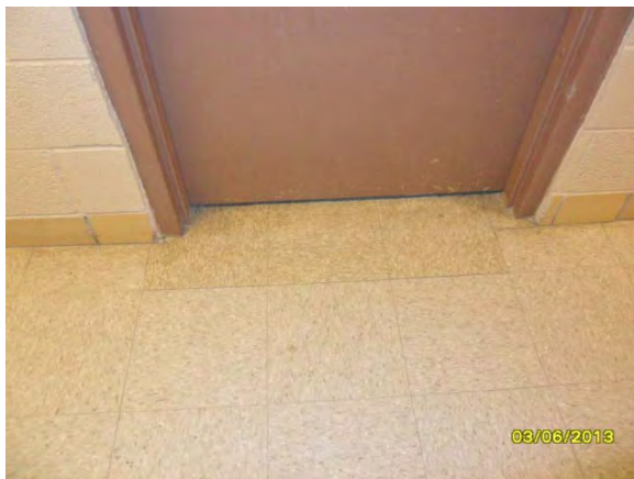
A-23. Administration Building, VCT Types Outside Utility Closet, Main Hallway Room 102, Outside Room 112.
