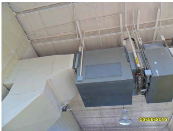
A-33. Administration Building, Assembly Hall, Room 120, Southwest HVAC Unit.
