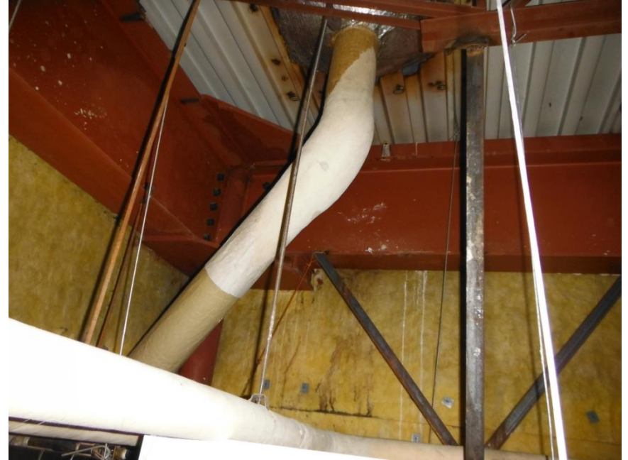
Photo 2. Typical asbestos-containing mudded roof drain
