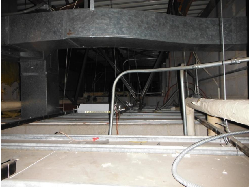
Photo 1. Typical asbestos-containing mudded elbow
